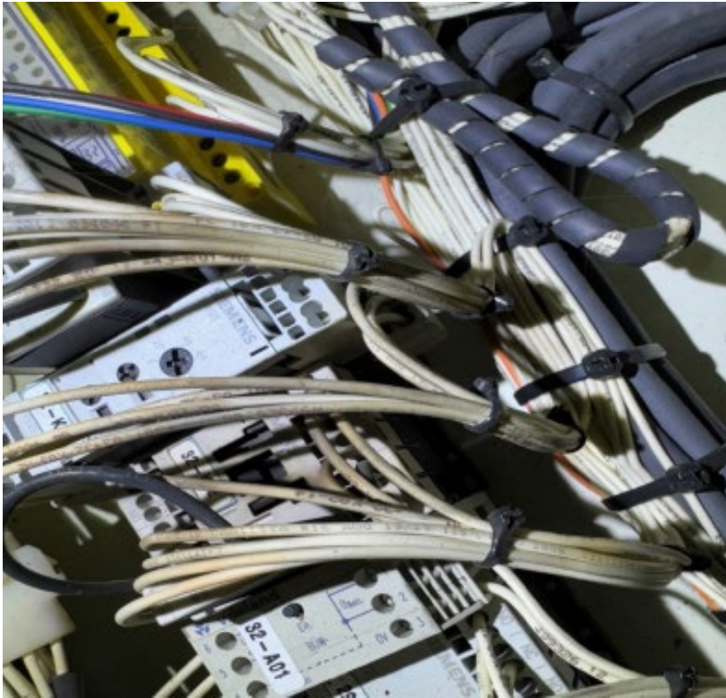
Damaged 32-K02 relay and wiring.
