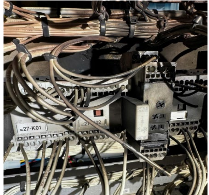
Damaged 32-K05 and 32-K06 relays and wiring.
