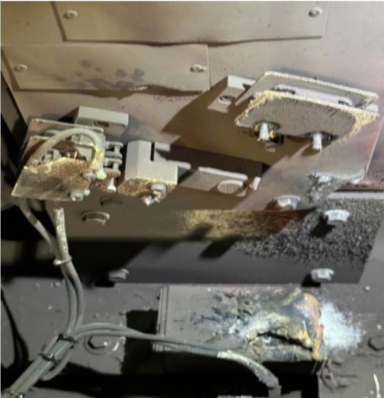
Main input fuse and back side of knife switch w/limit switches.
