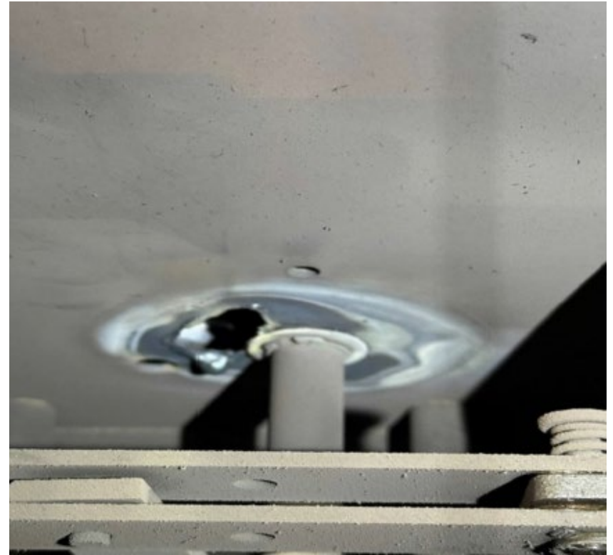
Damage to back side of shop power knife switch.
